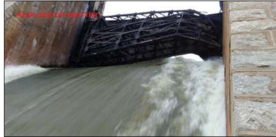
fig. 2 : Failure of Gate no 1 in Krishnagiri Dam
