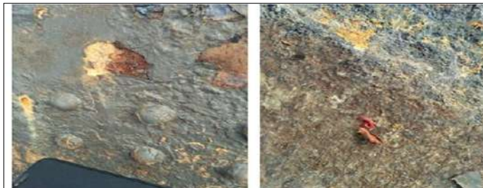
Fig. 3 : Corroded portion of the Gate no 1 in Krishnagiri Dam
