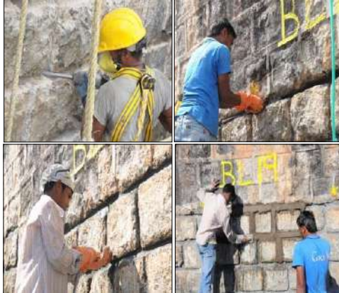
Fig.6: Execution of upstream face treatment (Racking, Cavity Filling, Injection Grouting and Raised Pointing)
