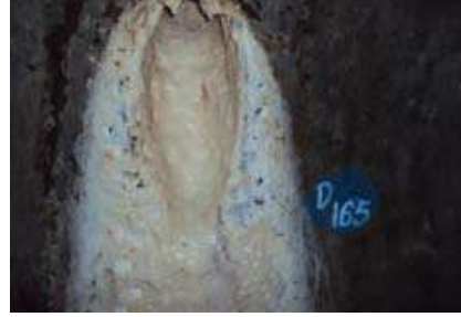
Fig. 3 : Leaching observed in drainage shaft
