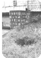
Figure 2. Formation of sinkhole
