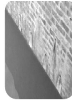
Figure 3. Weep Holes showing lime deposits
