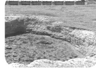
Figure 10. Superficial kankar strata on the reservoir bed
